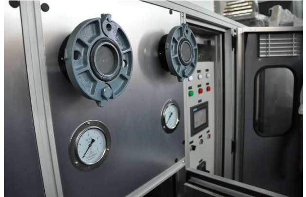
Inlet and outlet flanges of integrated AHU system
