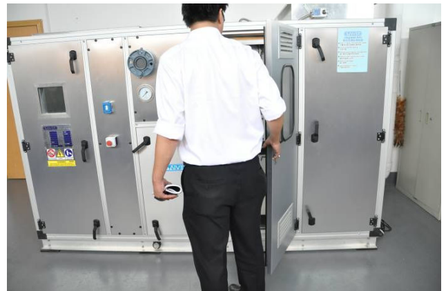
View of integrated AHU system
